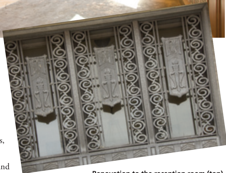
Renovation to the reception room (top) will restore it to its original look of the 1930s. Photo below shows extensive metalwork outside above the main entrance.
