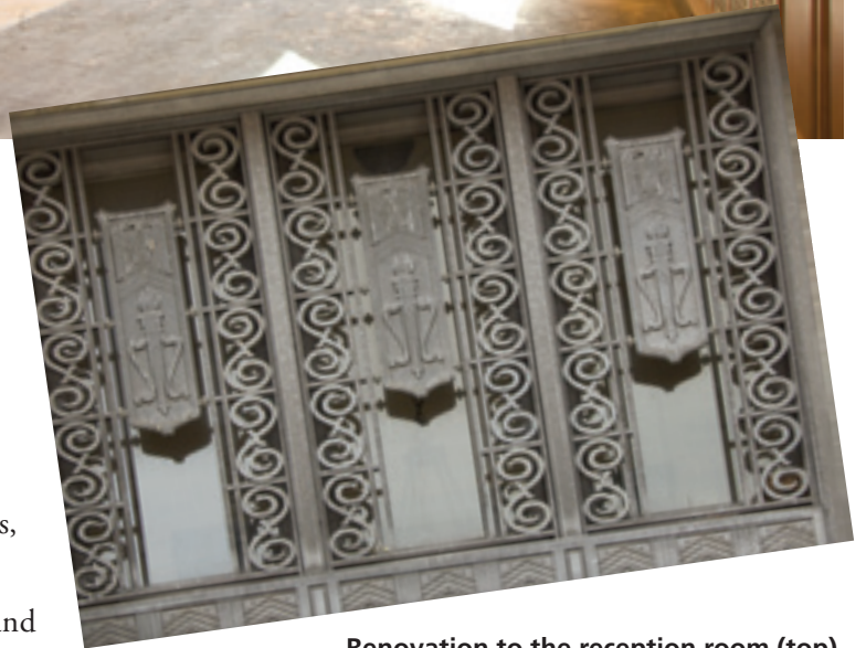
Renovation to the reception room (top) will restore it to its original look of the 1930s. Photo below shows extensive metalwork outside above the main entrance.
