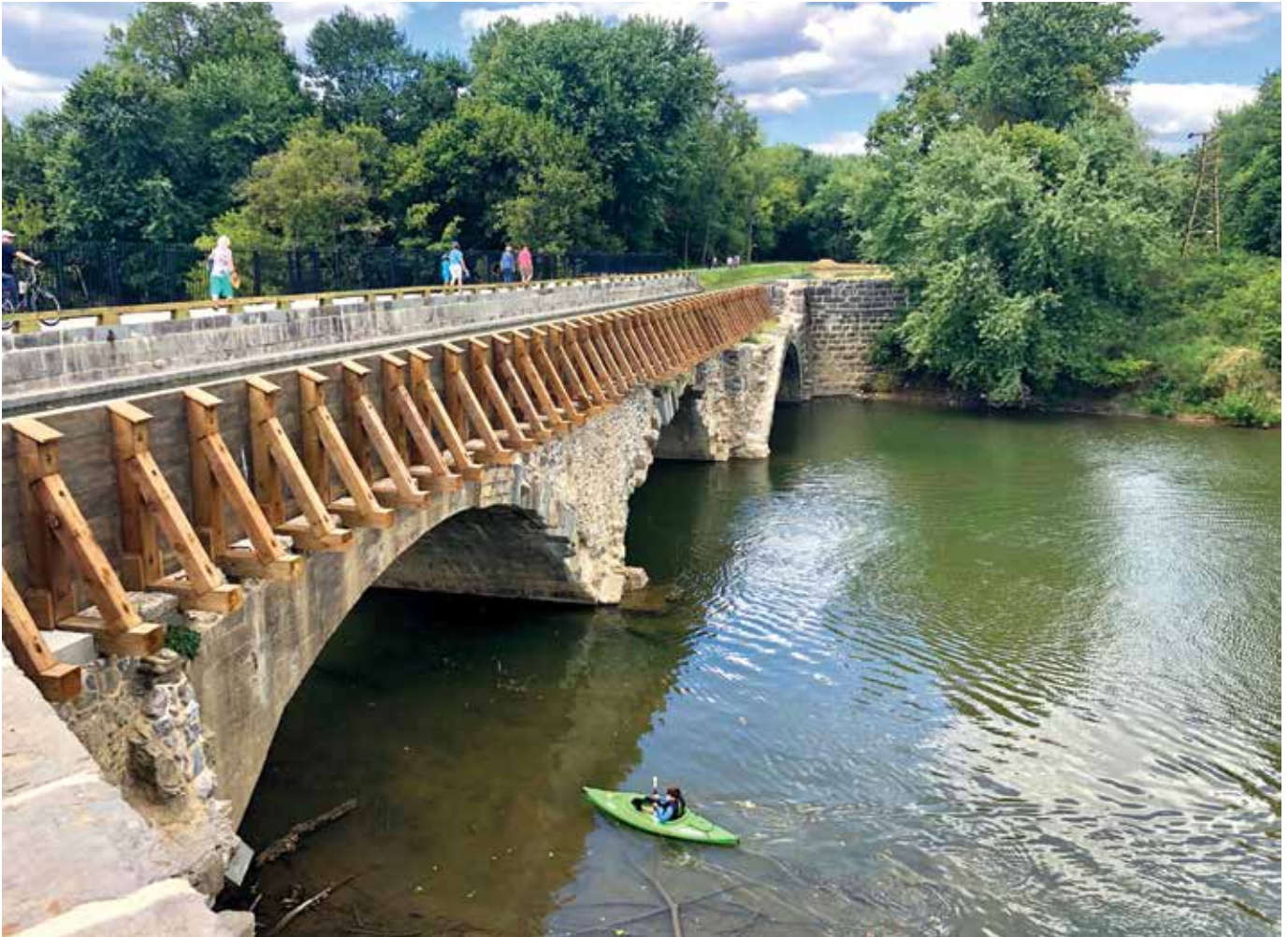
The Conococheague Aqueduct near the Cushwa Basin at Williamsport, MD, was a two-year restoration project between the National Park Service and the State of Maryland, making it possible for the aqueduct to again carry water. Visitors can take a canal boat tour across the aqueduct or they can paddle their own boat through the aqueduct or under it as shown in this photo. PHOTO BY DWIGHT WINGERT
